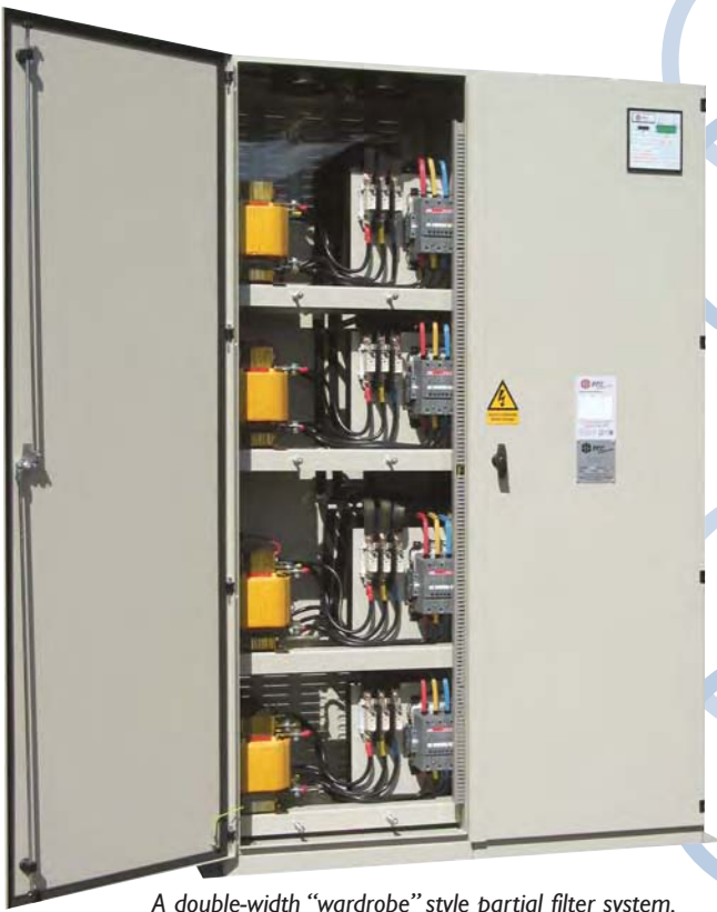
A double-width "wardrobe" style partial filter system. Cabling is accessed from above-right with this example
